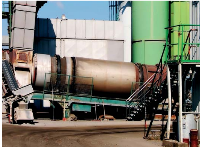
Application example: Rotary kiln within the chemical industry
